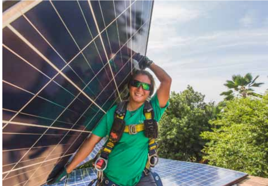
Technician installs rooftop solar system to boost residential energy efficiency. (Photo: SolarCity)
